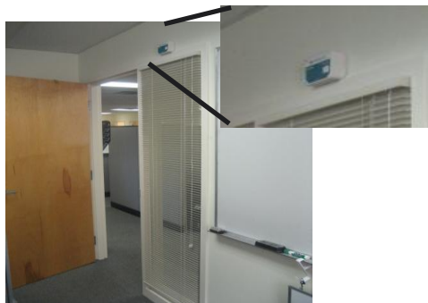
Figure 26: Example of Smart Sensor deployed in Commercial environment.
