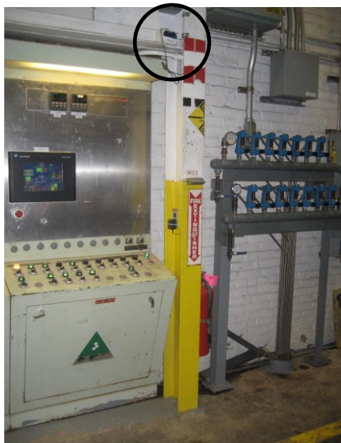
Figure 27: Example of Mesh Router placement in Light Industrial environment.
